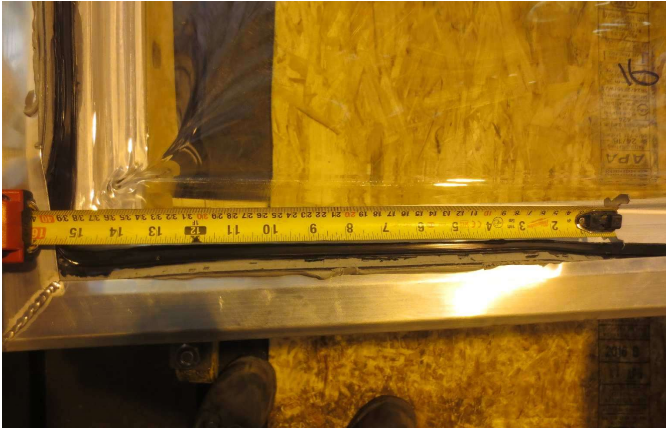
Picture 3 (Permanent deglazing at corner)
